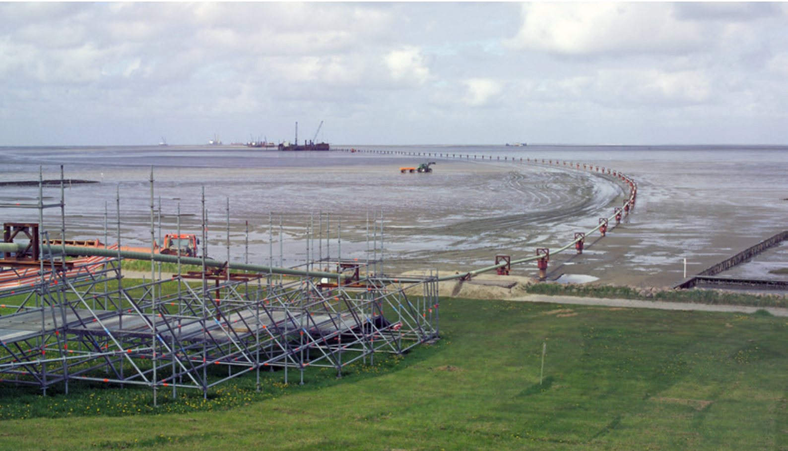
Duplex pipes for an offshore application in the North German Wadden Sea: transport of the pipelines using posts with roller bearings
